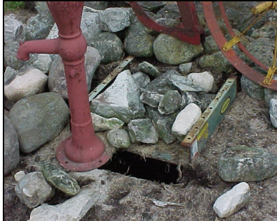
An old hand pump over a dug well.
