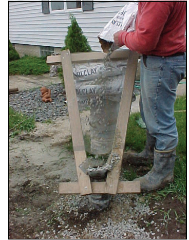
Well driller pouring bentonite chips into a drilled well to properly abandon the well.
